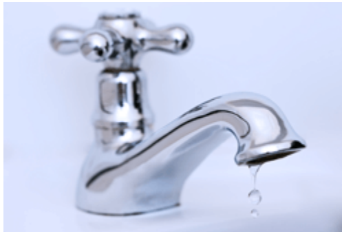
a leaking faucet
